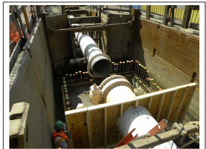
36" trunk main and valve installation at Furman Street and Old Fulton Street.
